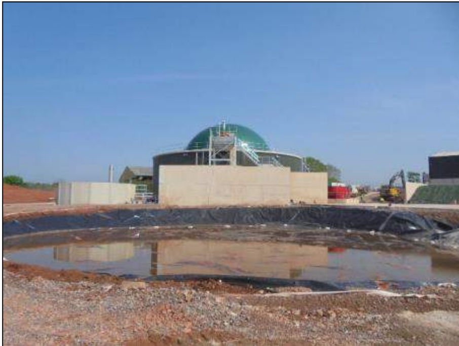
Photo 3-1 The excavated area for an additional feature of the proposed alterations to the site in the foreground, and the existing anaerobic digester and associated structures in the background. Taken from the south-east of the site looking west
